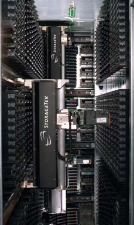
Interior photo of StorageTek SL8500 modular library system
